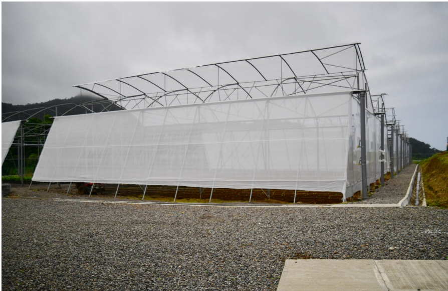
Greenhouse Park Facility at Montreal
